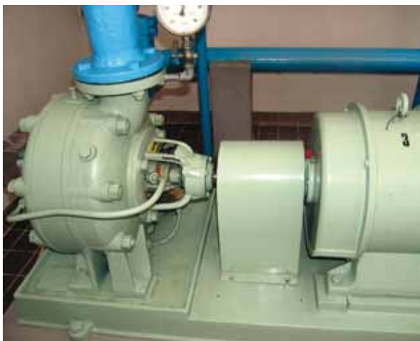
The pump runs today as master pump
