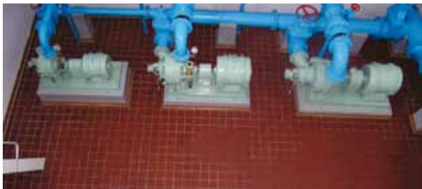
This pump is more than 70 years old and has run more than 560.000 hours!
