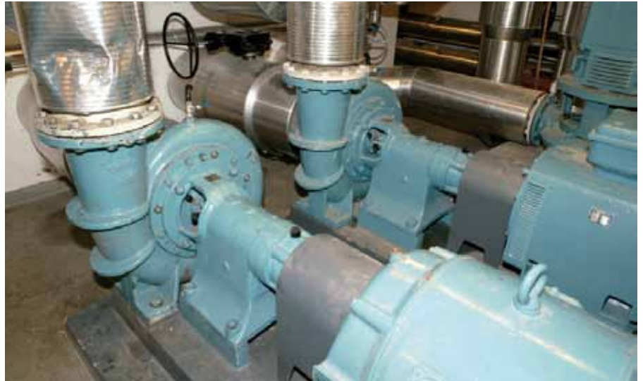
The Heating station in Horsens has in the past bought Trium pumps. They have now been in operation for about 40 years. The pumps have up to now been in service without any problems.
